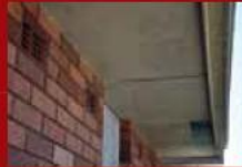
Unsecure eave joints
