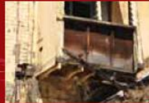
Exposed asbestos after a fire
