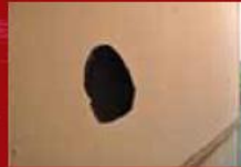
Holes in fibro walls
