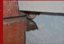
Damaged Tilux in bathrooms or laundries
