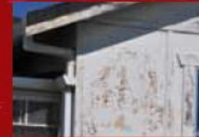
Exposed asbestos due to peeling paint
