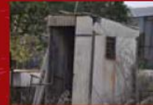
Falling down outhouses
