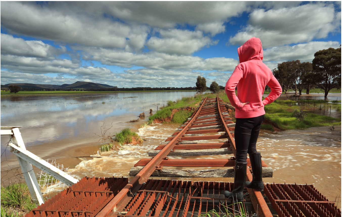
Floodwaters and the buckled train tracks at Crowther, Hilltops Region, New South Wales.
