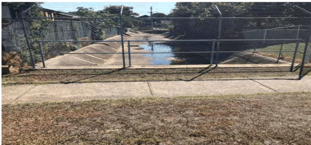
Figure 10: Existing Open Concrete Stormwater Channel Between Cumberland Road and Palmer Street (to be Culverted)
