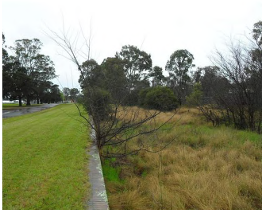
Figure 4 HR-1 looking north: railway embankment at right of picture and cut-off wall to the left
