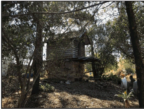
Figure 21. View of dilapidated outbuilding to the west of the residential dwelling.
