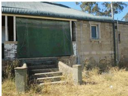
Figure 25: View of the north-west façade of Woodcrest, showing steps to the verandah.
