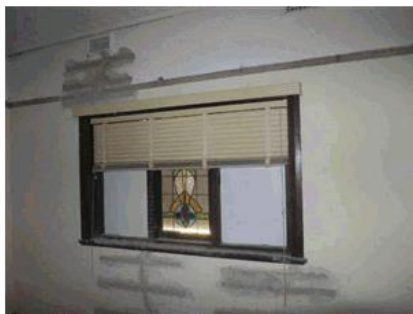
Figure 37: Windows facing the verandah, now boarded up after theft of stained glass casements.
