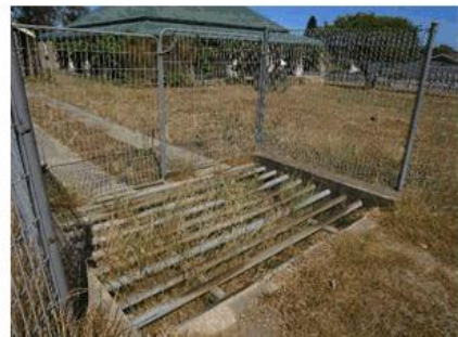
Figure 20: The cattle grid on the driveway of the subject site, accessed from Oxford Road.
