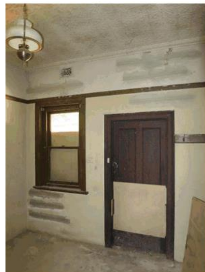
Figure 40: View of the rear room, showing the pressed metal ceiling, concrete floor and recent structural work to walls.
