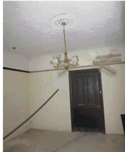
Figure 36: View of a bedroom, showing the pressed metal ceiling, concrete floor and recent structural work to walls.
