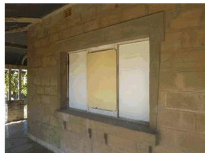
Figure 32: Boarded window on the north-east façade of the house, showing the home-made concrete blocks and rendered architrave and sill.
