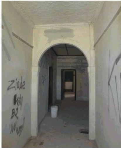
Figure 35: View of the hallway, facing south-west towards the lounge room and kitchen.
