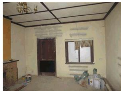
Figure 38: View of the lounge room, facing north-west, showing the fireplace and recent structural works to walls.
