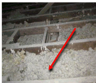
2. Friable (Loose) Asbestos based loose-fill insulation
