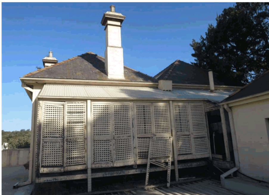
Figure 23 – The rear veranda is from the 1985–95 period. It screens the air-conditioning equipment. NBRSArchitecture February 2017.
