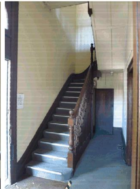
Figure 30 – The original stair, with more recent carpet and stays, in G.04. NBRSArchitecture February 2017.
