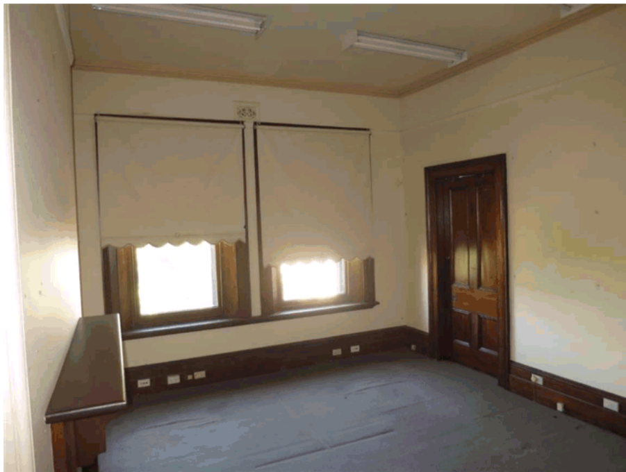
Figure 34 – Room F.04 has original skirting, window, door and cornice. Later services have been cut into the, and mounted onto, the timber skirting. NBRSArchitecture February 2017.
