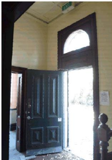
Figure 29 – The original door to the residence on the south-west side, original cornice. The splayed trim at the bottom of the leaf is not original.
