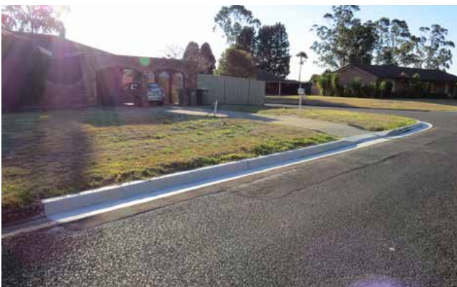
Kerb and gutter along with layback at Dandenong Crescent, Ruse after reconstruction
