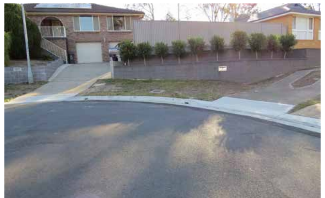
Kerb and gutter along with layback at Yulunga Place, Bradbury after reconstruction
