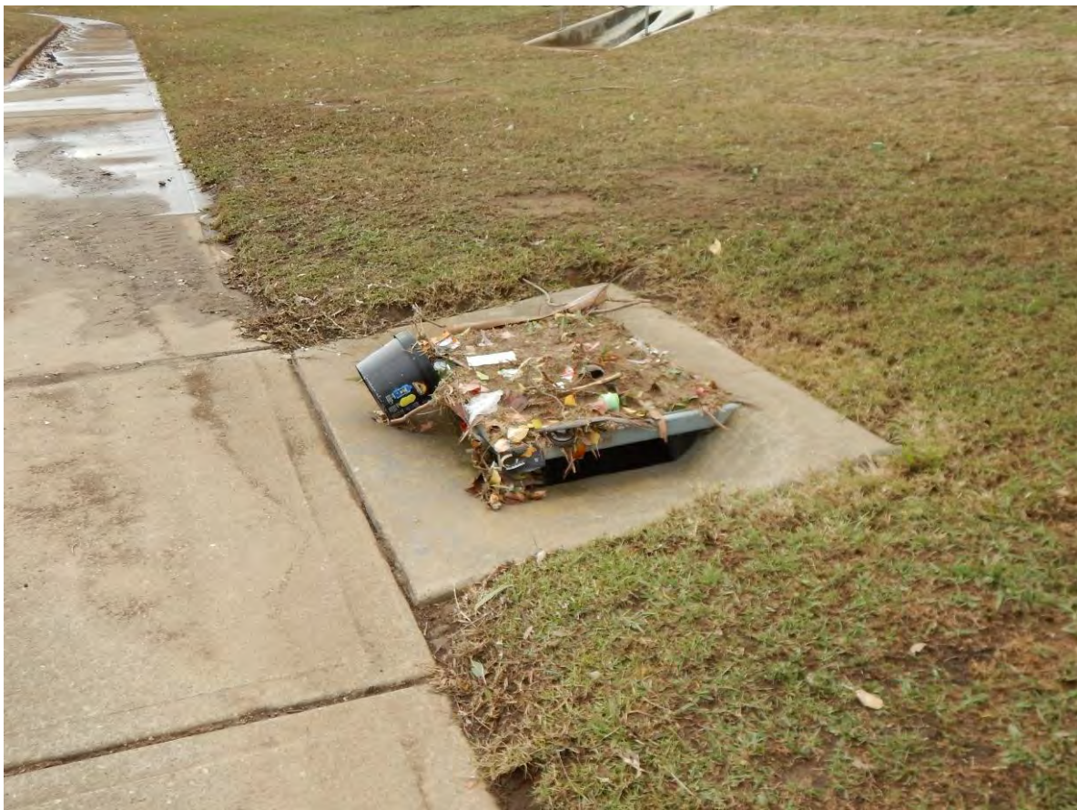
Plate 10 Example of blockage of stormwater pit at Oswald Reserve, St Helens Park
