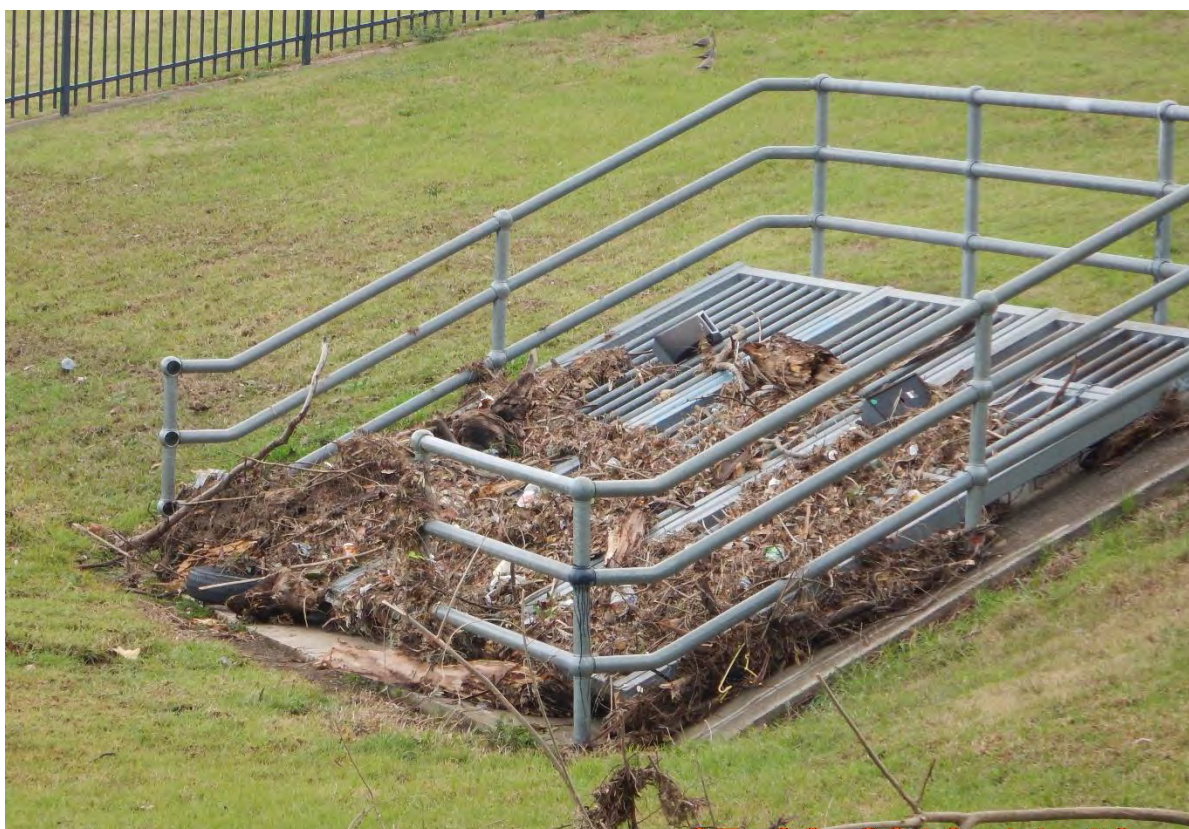
Plate 9 Example of blockage of culvert following a rainfall event
