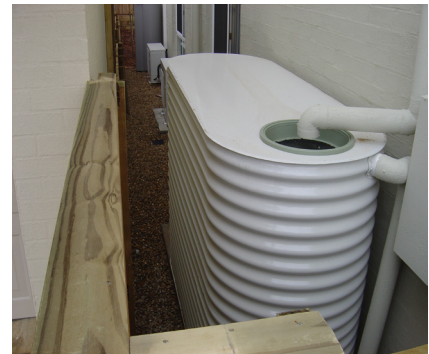
Figure 2.4.1 - An example of a domestic rainwater tank.
