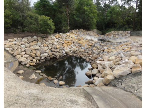
Figure 2.10.2 - Water quality devices can improve water quality and give an important visual enhancement to a development area.
