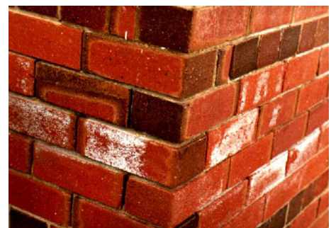
Figure 2.14.1 - Salt damage in the brickwork of buildings identifies a possible salinity problem in the area.
