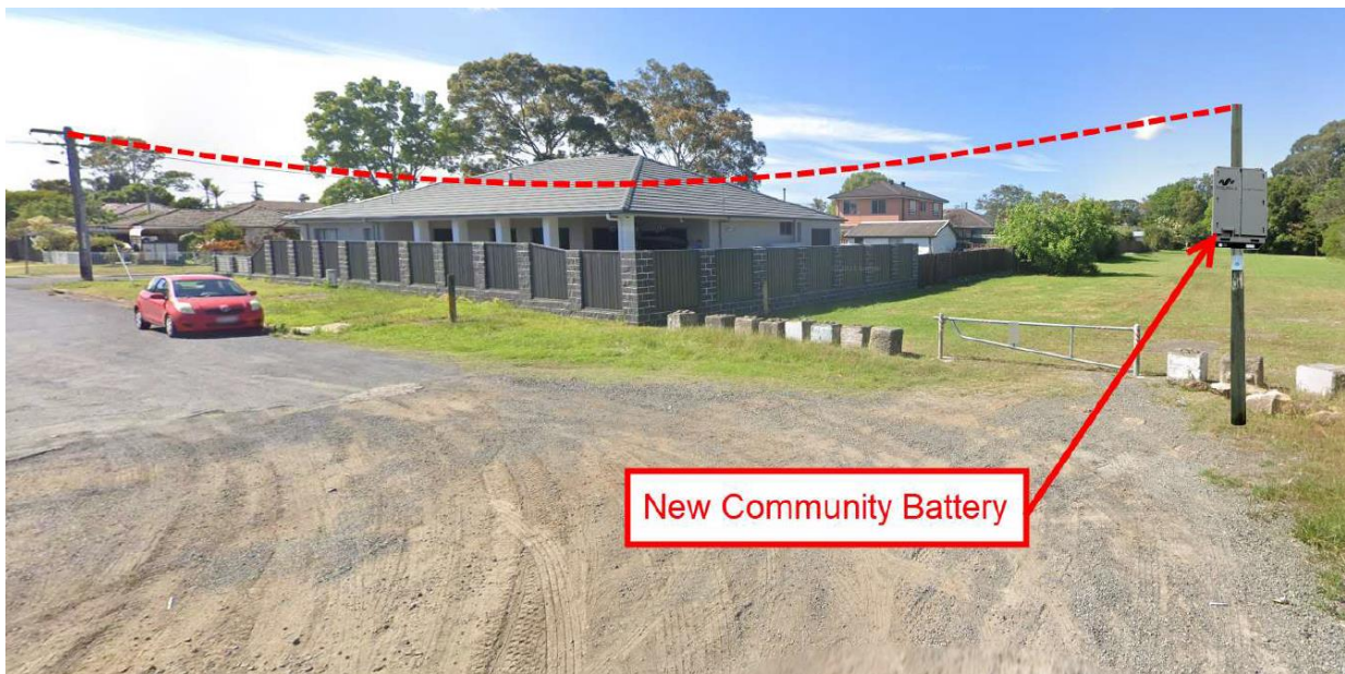
Figure 1: Pole mounted community battery at Railway Parade, Macquarie Fields
