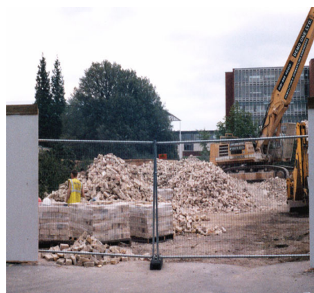
Figure 2.9.1 - Demolition waste materials separated and stored on-site until they are safely removed for reuse, recycling or disposal.
