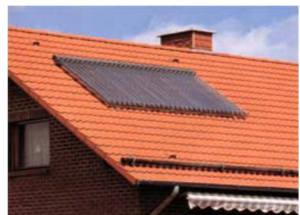
Figure 2.4.2 - Solar hot water panels facing north.
